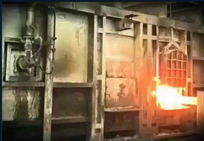
Billet furnace in operation
